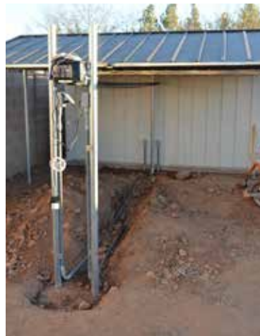
Figure 29: Supports and Conduit for the Garage Door Opener
