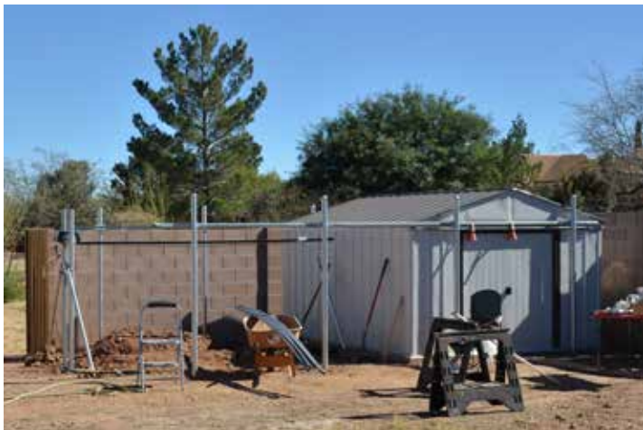
Figure 28: Modified Aero Shed Roll-Off Observatory with Partially Complete Roof Tracks and Opener
